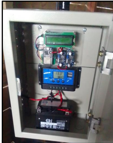
Gambar 4.3 Box Panel Alat control
