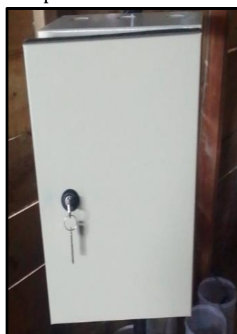
Gambar 4.2 Box Panel Control
