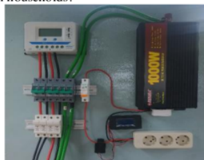
Fig 13. Off-Grid System Device
